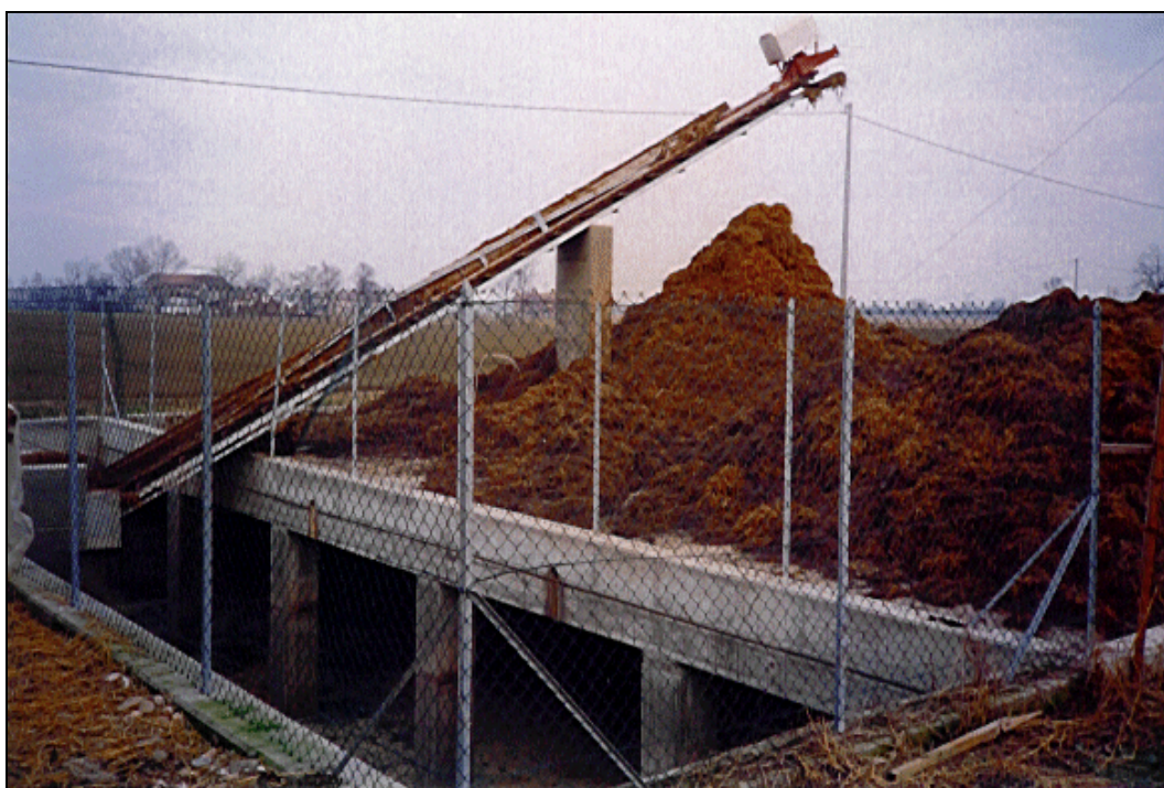
Figure 2.33: Storage of littered manure with separate containment of the liquid fraction (Italy)
